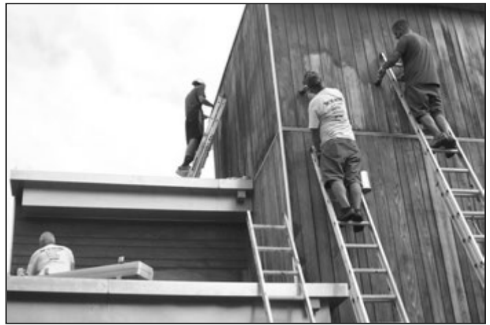
A crew from Top to Bottom Painting and Renovations spent hours cleaning and staining the exterior of the Parish Center.
